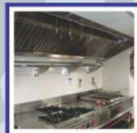
Kitchen Hood Fire Suppression Systems
